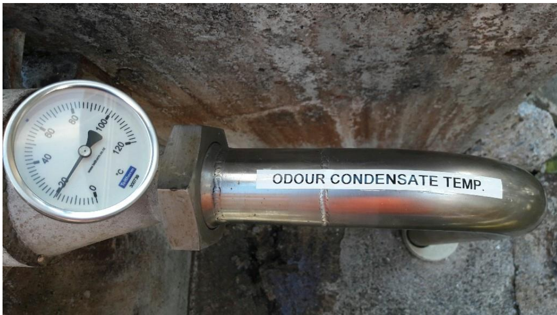
Odour Condensate Temperature Gauge
