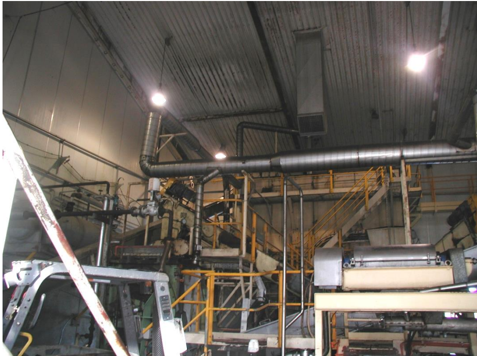
Wetside Extraction Ducting – above Inside Raw Material Bin
