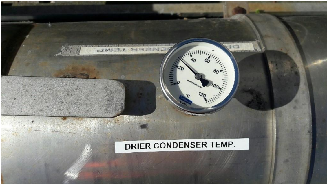
Drier Condenser Temperature Gauge
