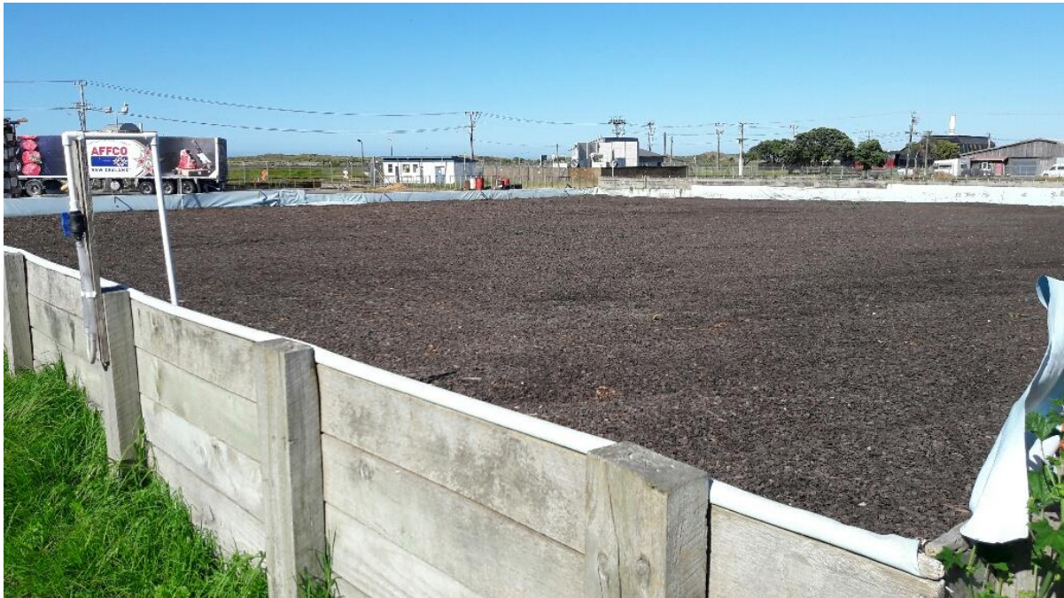
View of Main Bio Filter (looking South)
