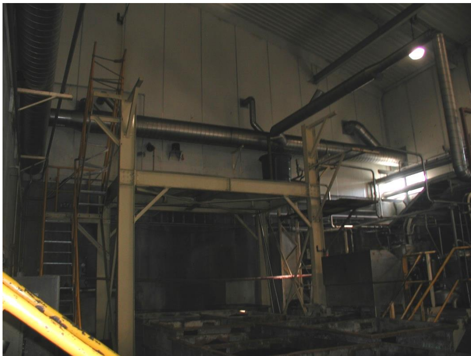
Wetside Extraction Ducting – exiting building to Wetside Cooling Tower
