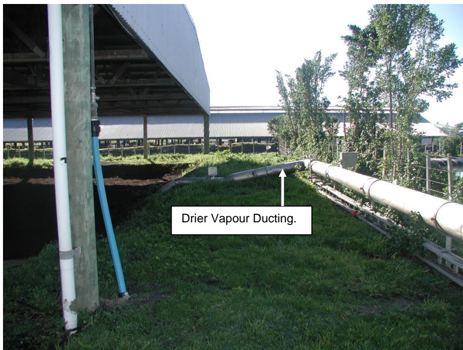
Drier Vapour Ducting entering Drier Bio Filter
