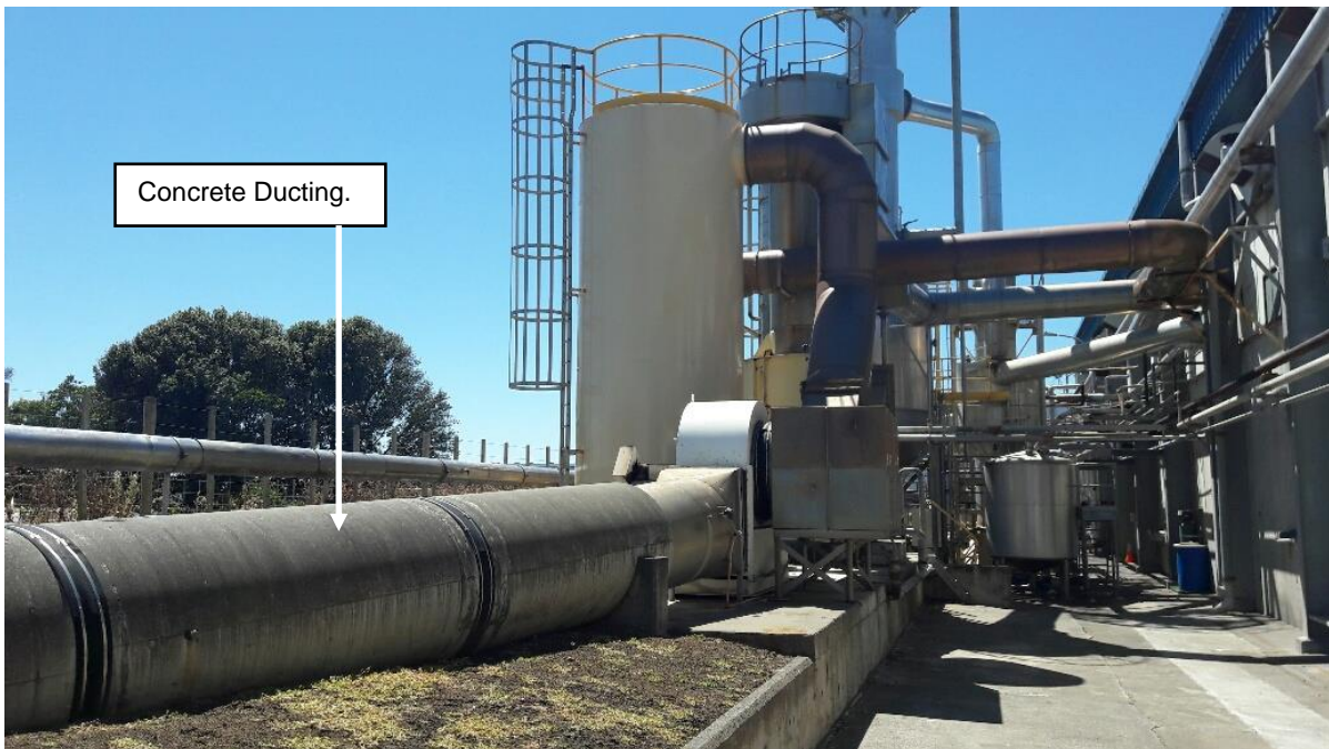
Concrete Extraction Ducting to Main Bio Filter
