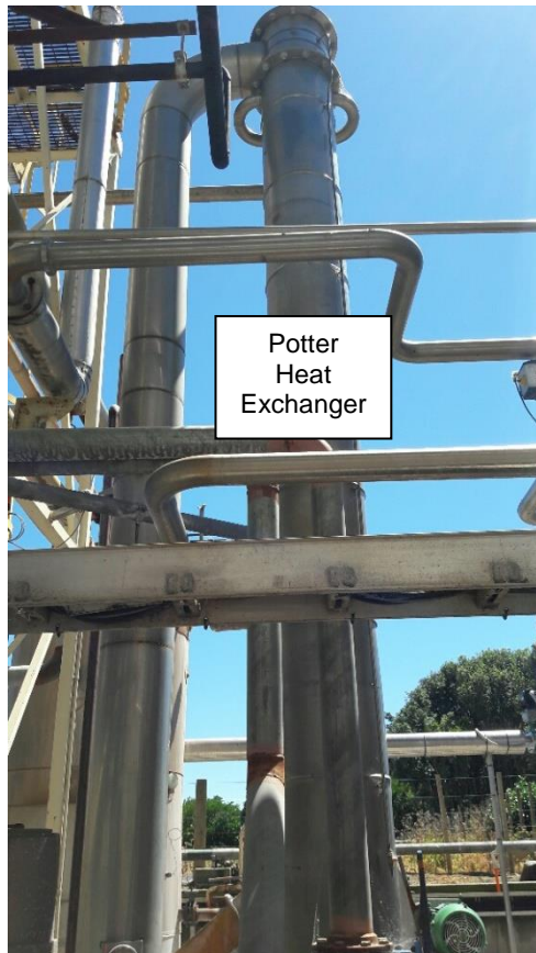
Dryside Vapours to Potter Heat Exchanger
