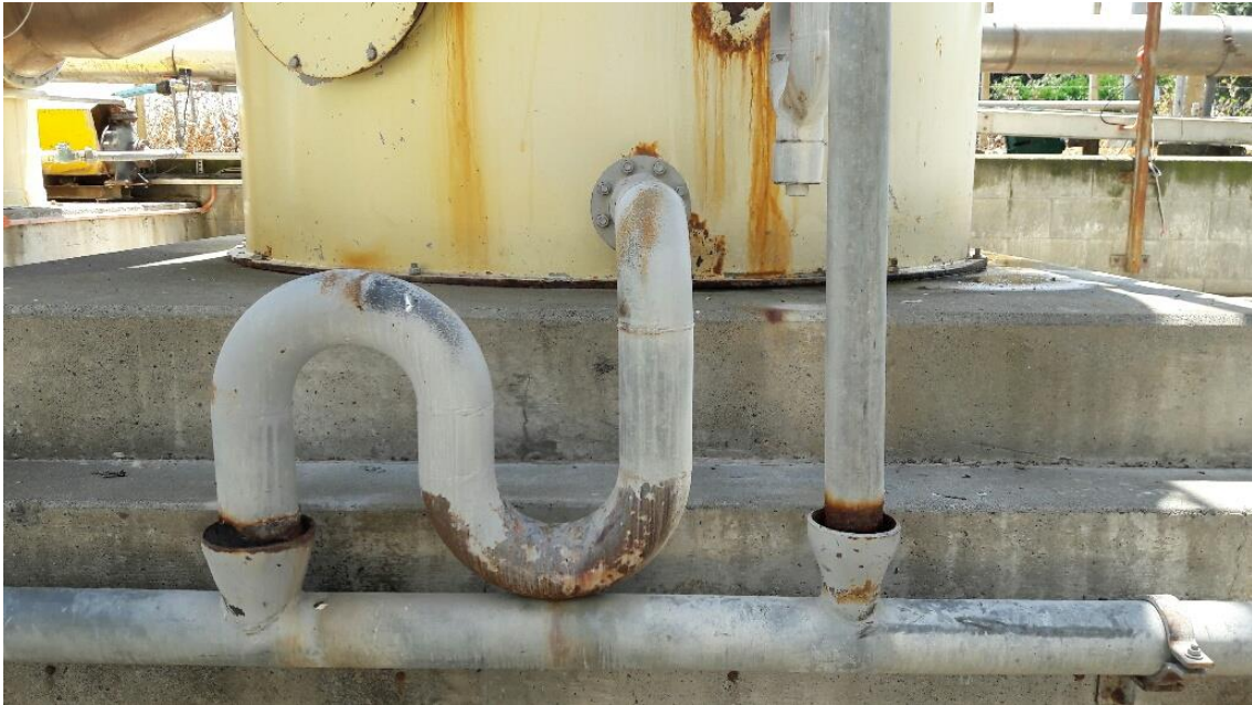
Wetside Cooling Tower Condensate Outlet
