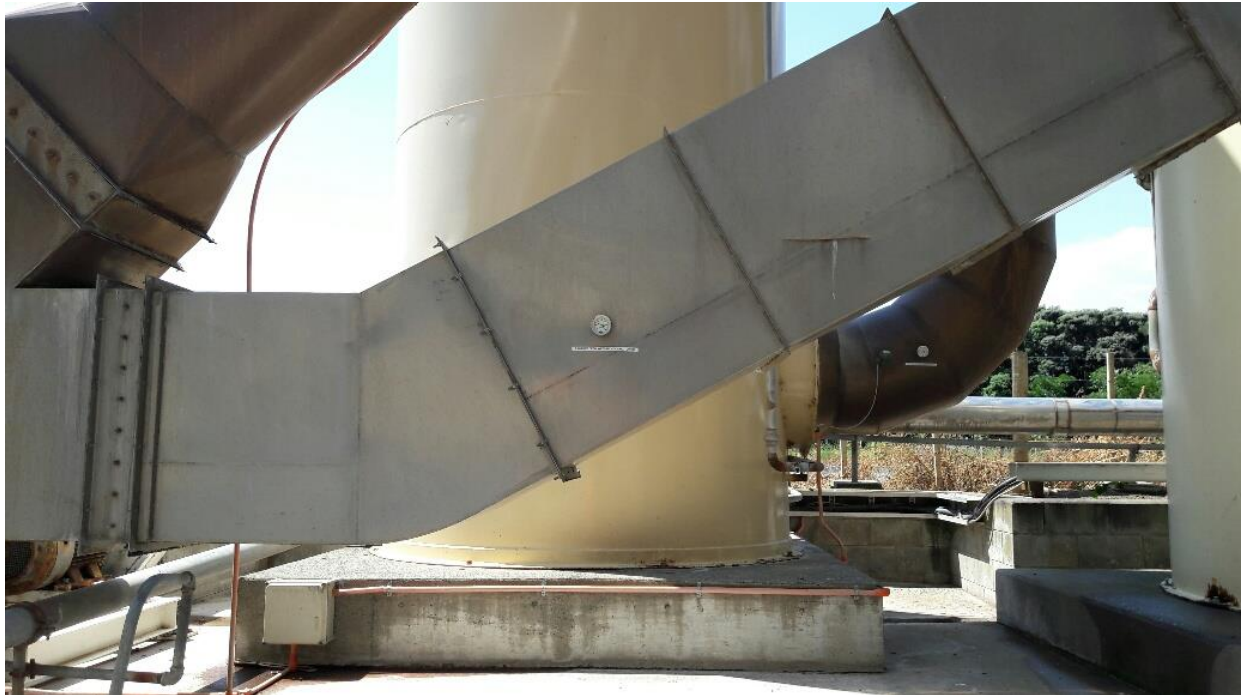
Exhaust from Wetside Cooling Tower (Manual Temperature Gauge)
