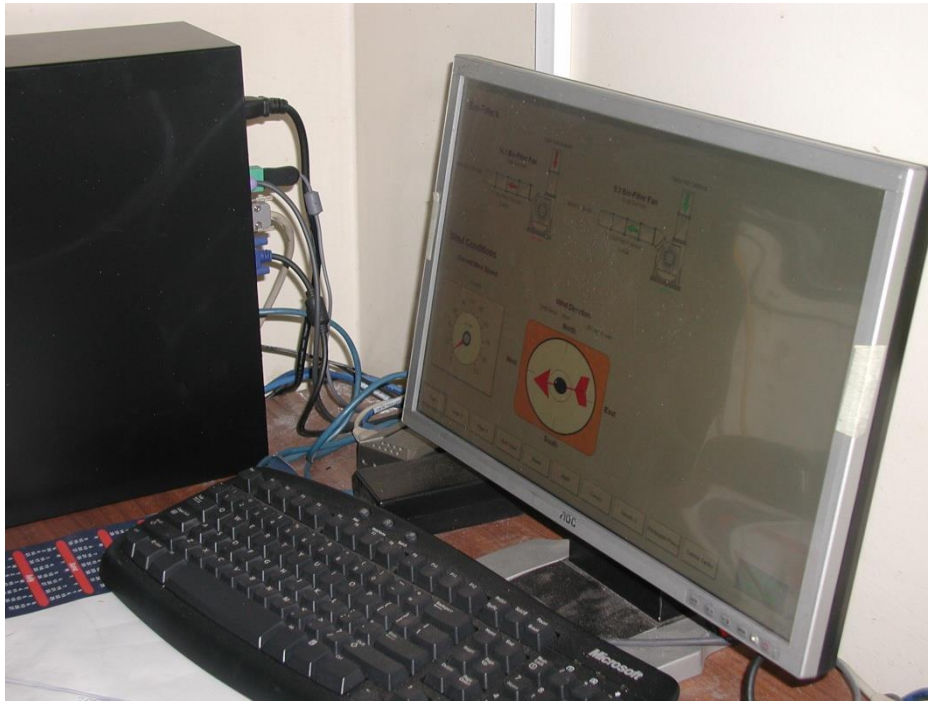
SCADA System – Continuous Monitoring of Consent Conditions
