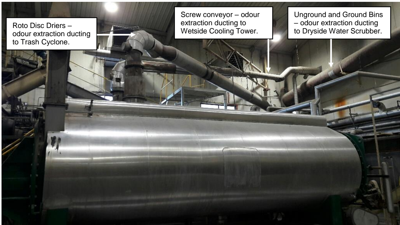
Dryside Extraction Ducting – exiting building to Trash Cyclone, Dryside Water Cooling Scrubber and Wetside Cooling Tower
