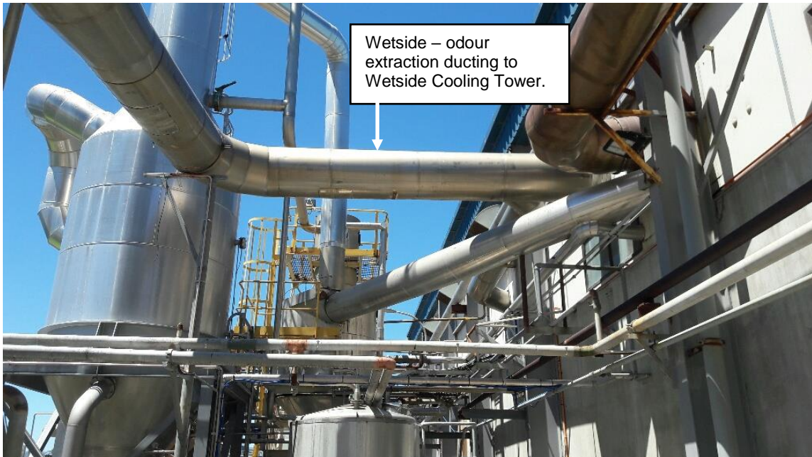
Wetside Extraction Ducting Exiting Building
