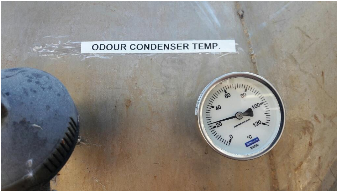
Location of Odour Condenser Temperature Gauge
