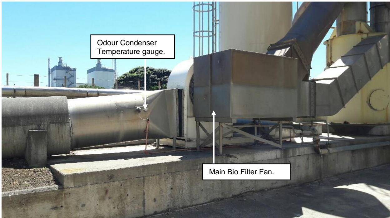
Exhaust from Main Bio Filter Fan to Main Bio Filter
