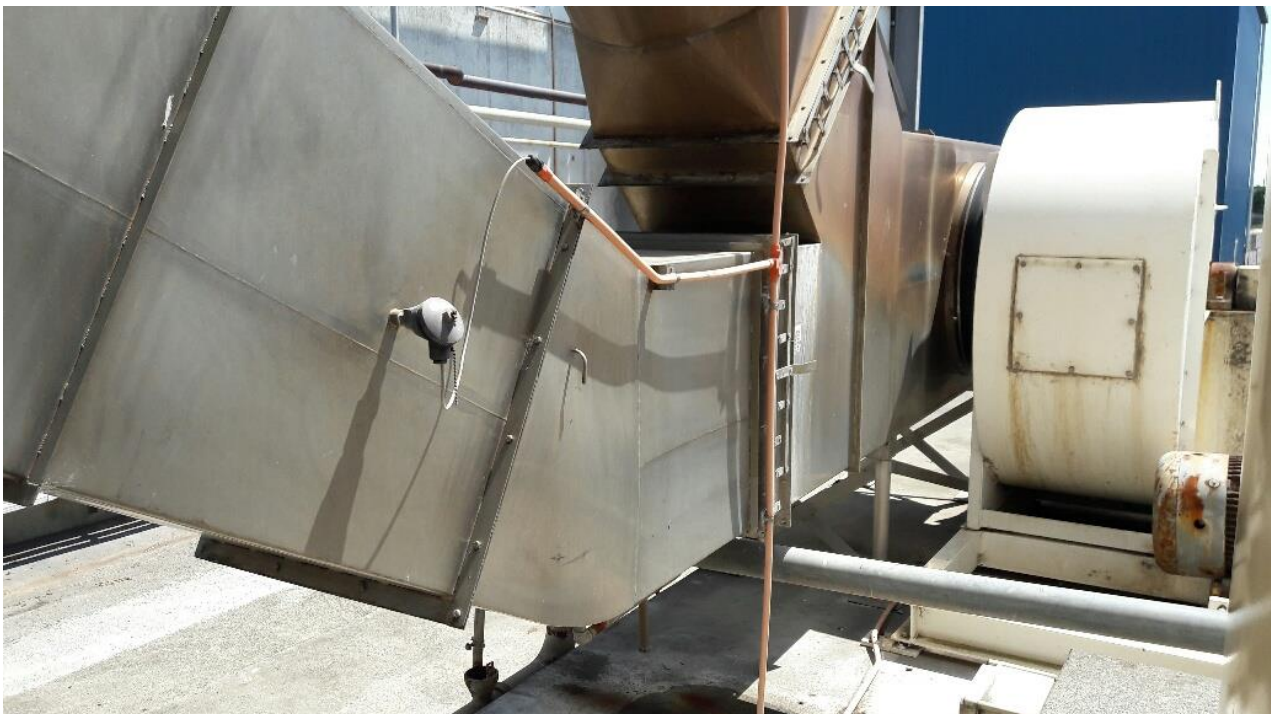
Exhaust from Wetside Cooling Tower – Transmitter:- Temperature (HRT4)
