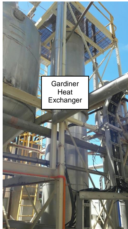
Vapours to Gardiner Heat Exchanger
