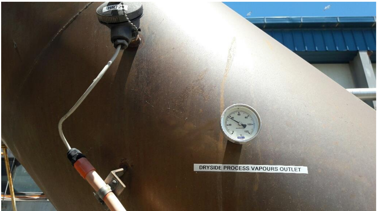
Dryside Water Scrubber Exhaust Outlet – Transmitter (HRT2) to Main Bio Filter Extraction Fan
